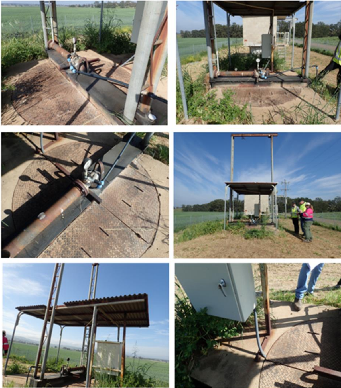
Figure 7 - Coolah Back -up Well
