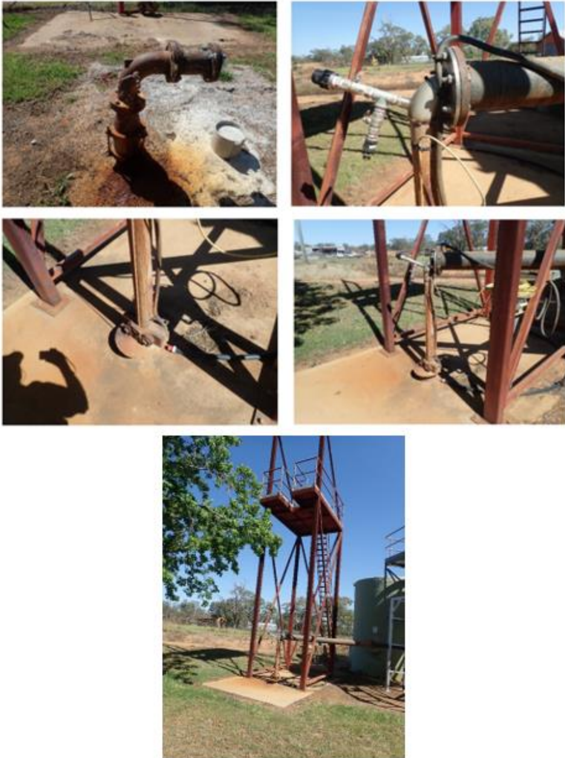
Figure 10 - Baradine Main Supply Bore
